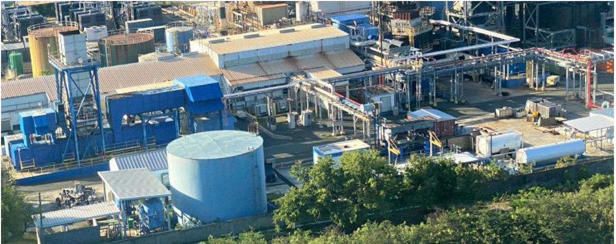
Figure 10. LPG Terminal at Estate Richmond Power Plant, St. Croix
